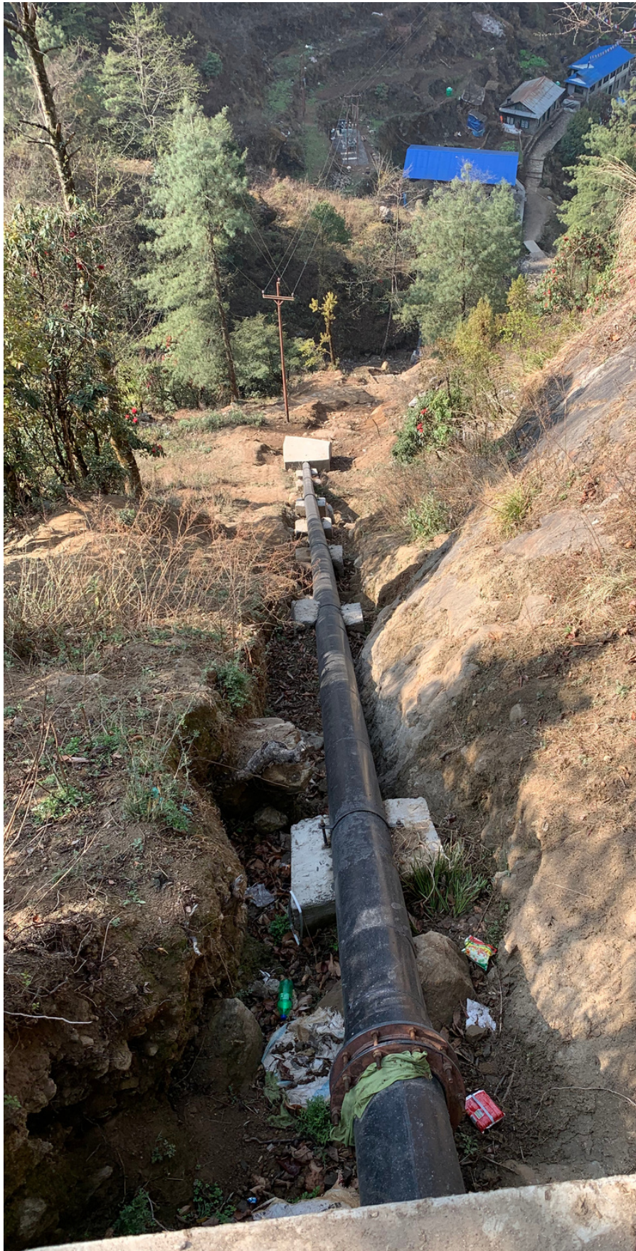
Hydro-pipes below Lukla
